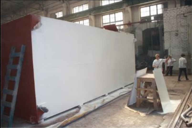
Thermal insulation of technological equipment supplied to various ships at the shipyard
