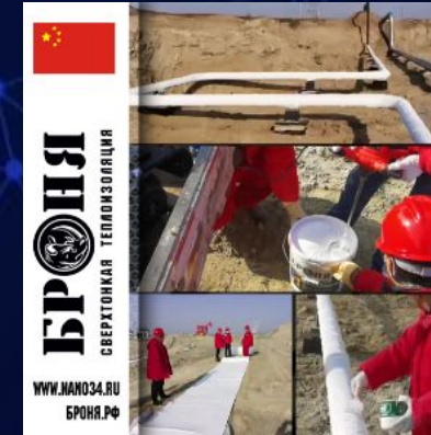
The start of the global application of the BRONYA Classic on the pipeline of the Klamas oil field of Shinjiang, China
