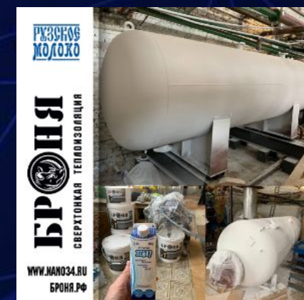
BRONYA Classic NF on hot water boilers of JSC "Ruz milk", Moscow region
